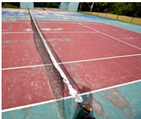
Tennis court cracks triggered a test case over liability insurance coverage.
